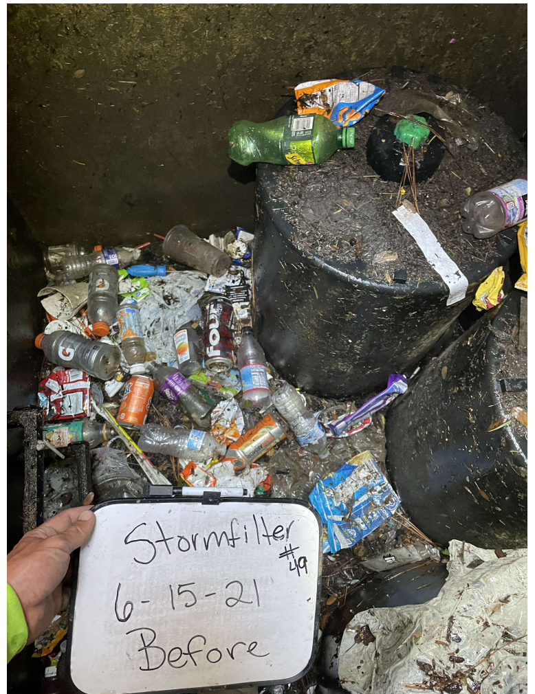
B49 Stormfilter Before
