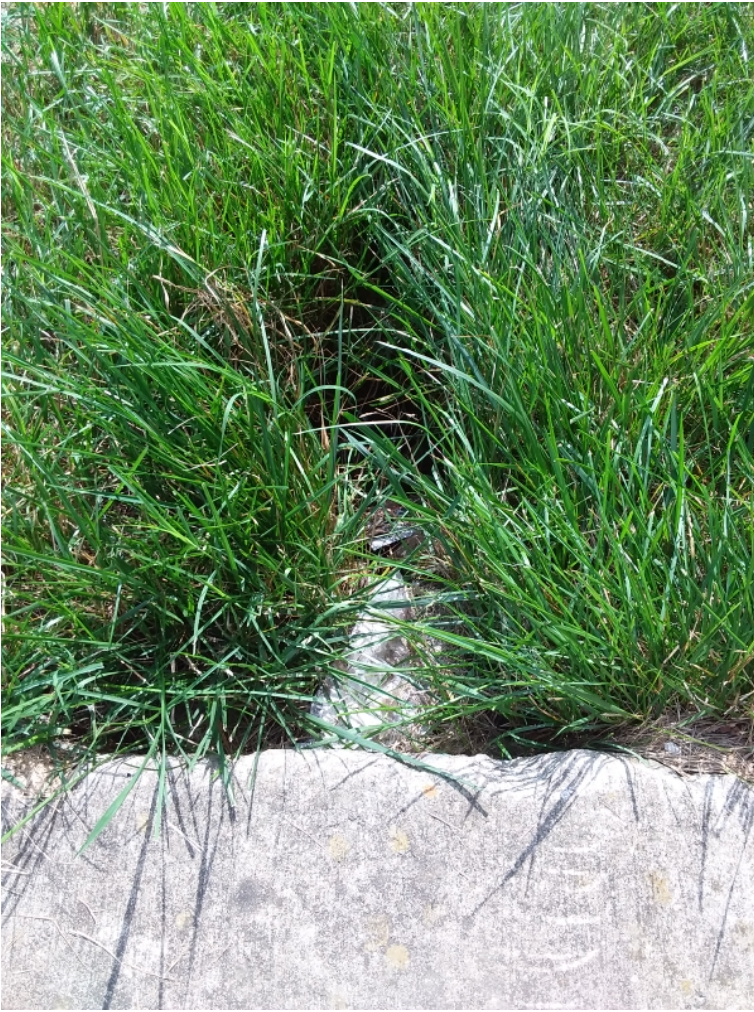
Noticed erosion and washout located SW of BMP 43
