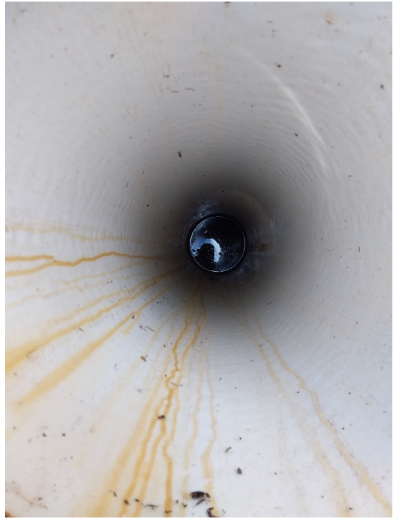
BMP 36: 16" of water standing in maintenance port
