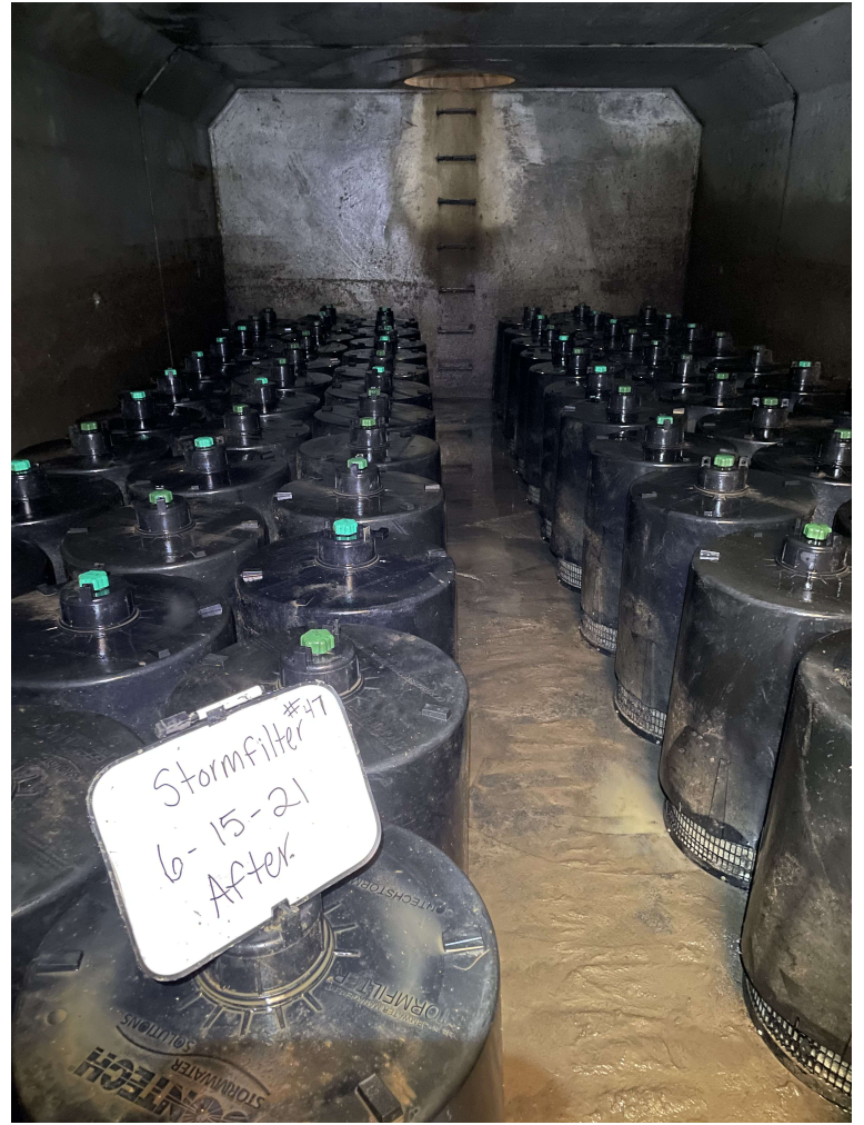
BMP 47 Stormfilter After
