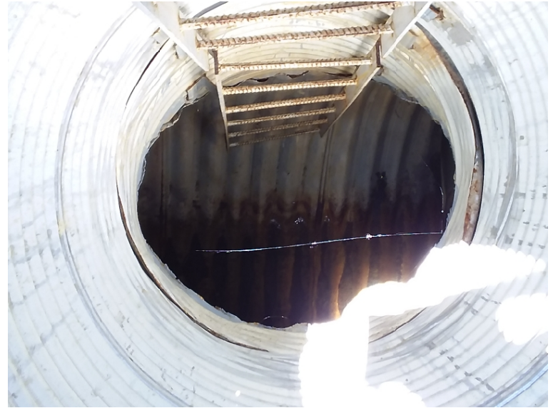
BMP 50- trace amounts of sediment
