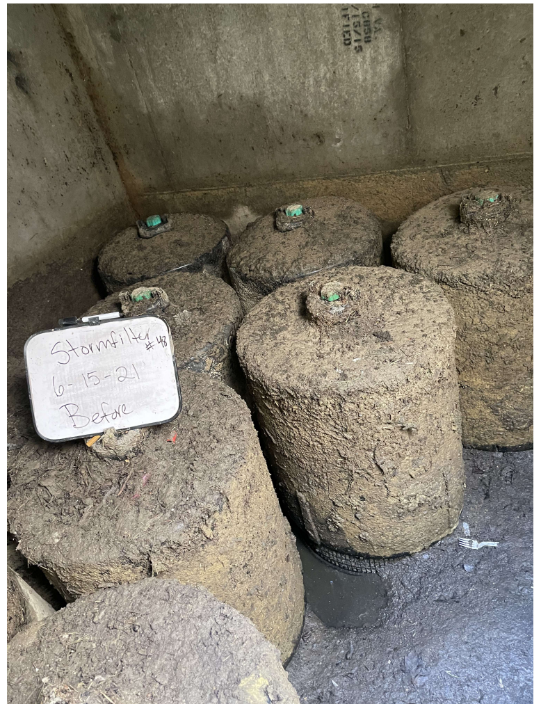
BMP 48 Stormfilter Before
