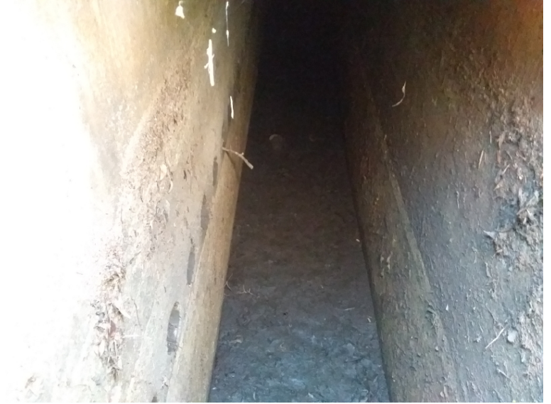
BMP 31: sediment chamber side- very little accumulation
