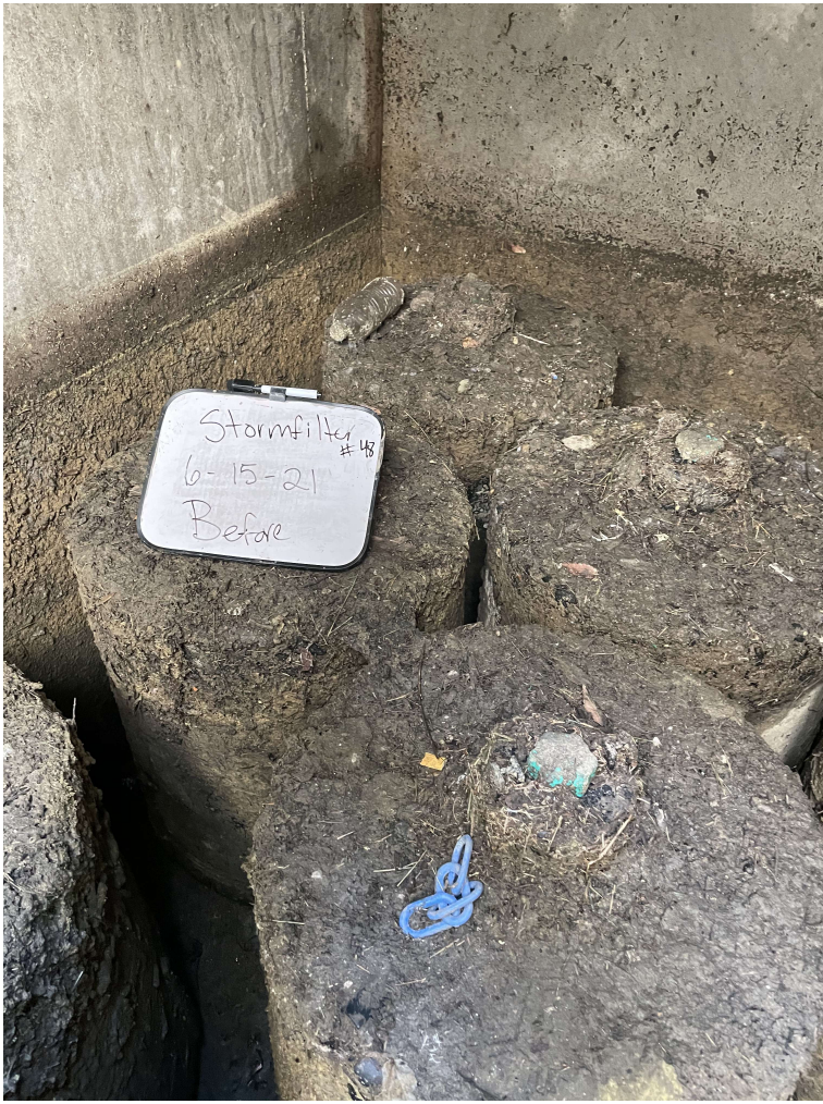
BMP 48 Stormfilter Before
