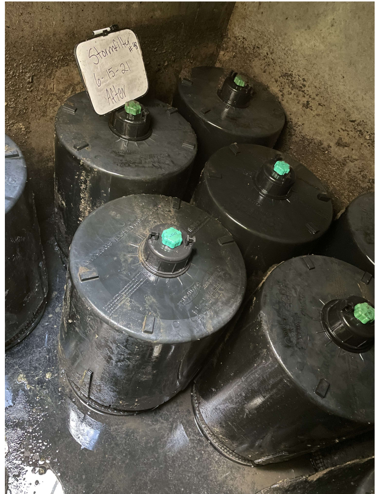
BMP 48 Stormfilter After
