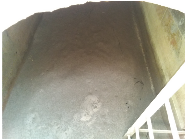
BMP 28- remove 3" of sediment accumulation from that is on top of fabric layer
