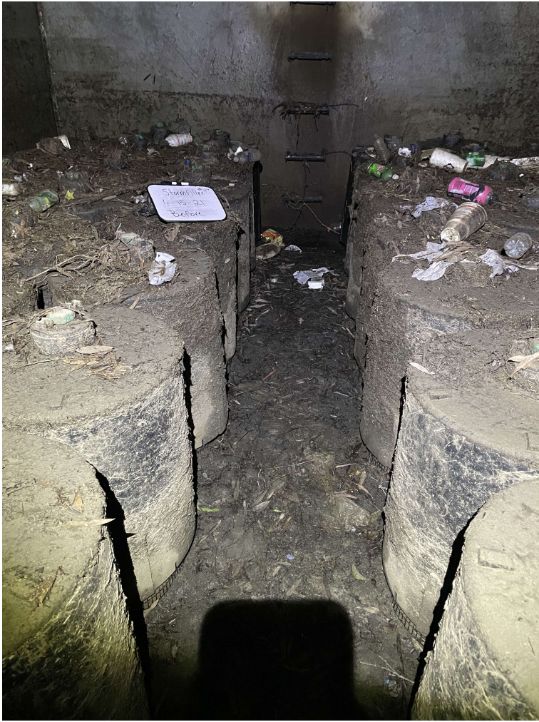
BMP 47 Stormfilter Before
