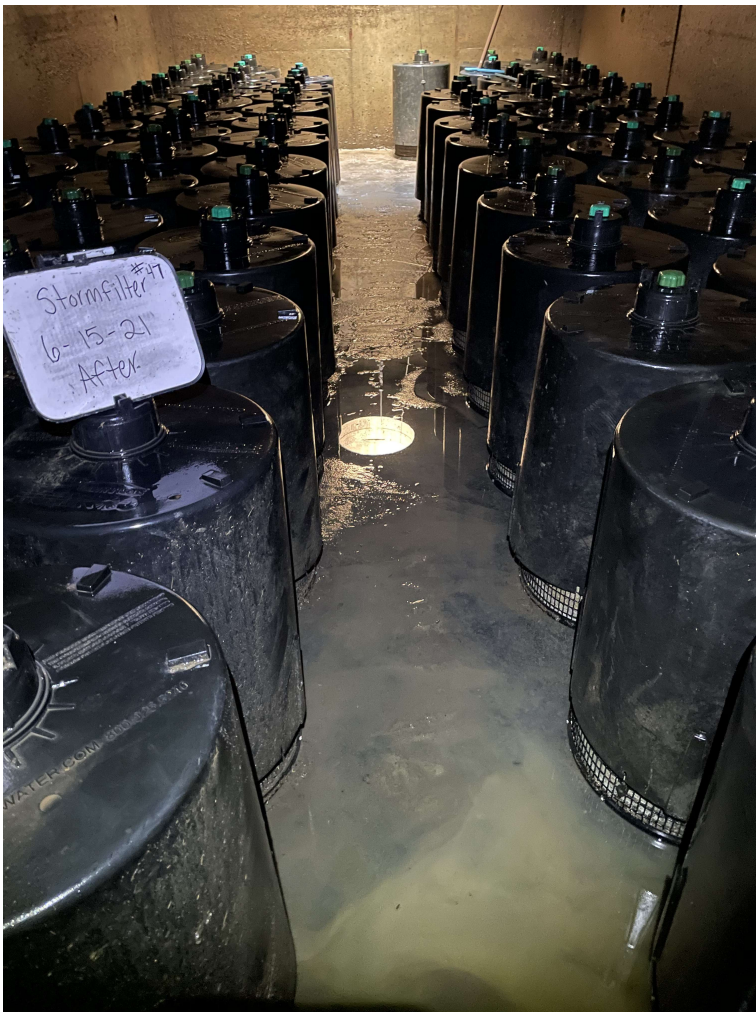
BMP 47 Stormfilter After
