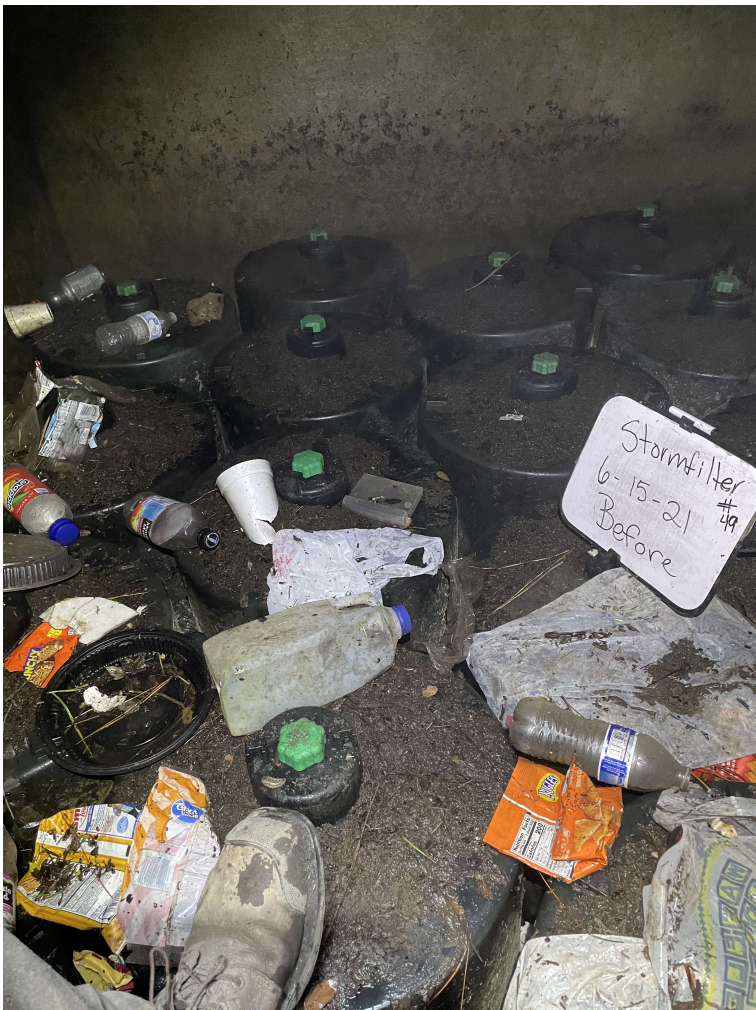
BMP 49 Stormfilter Before
