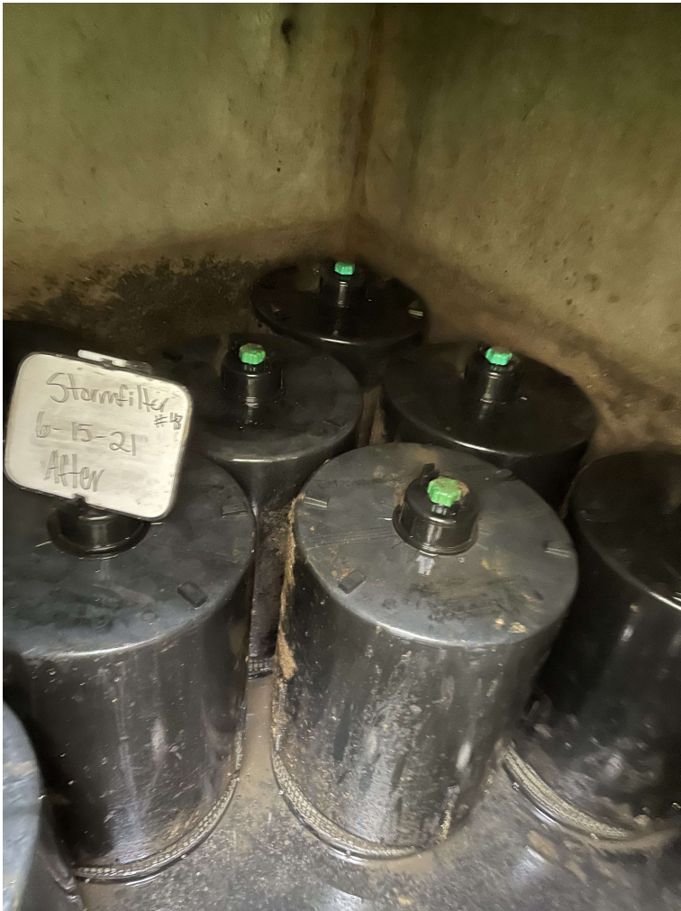
BMP 48 Stormfilter After
