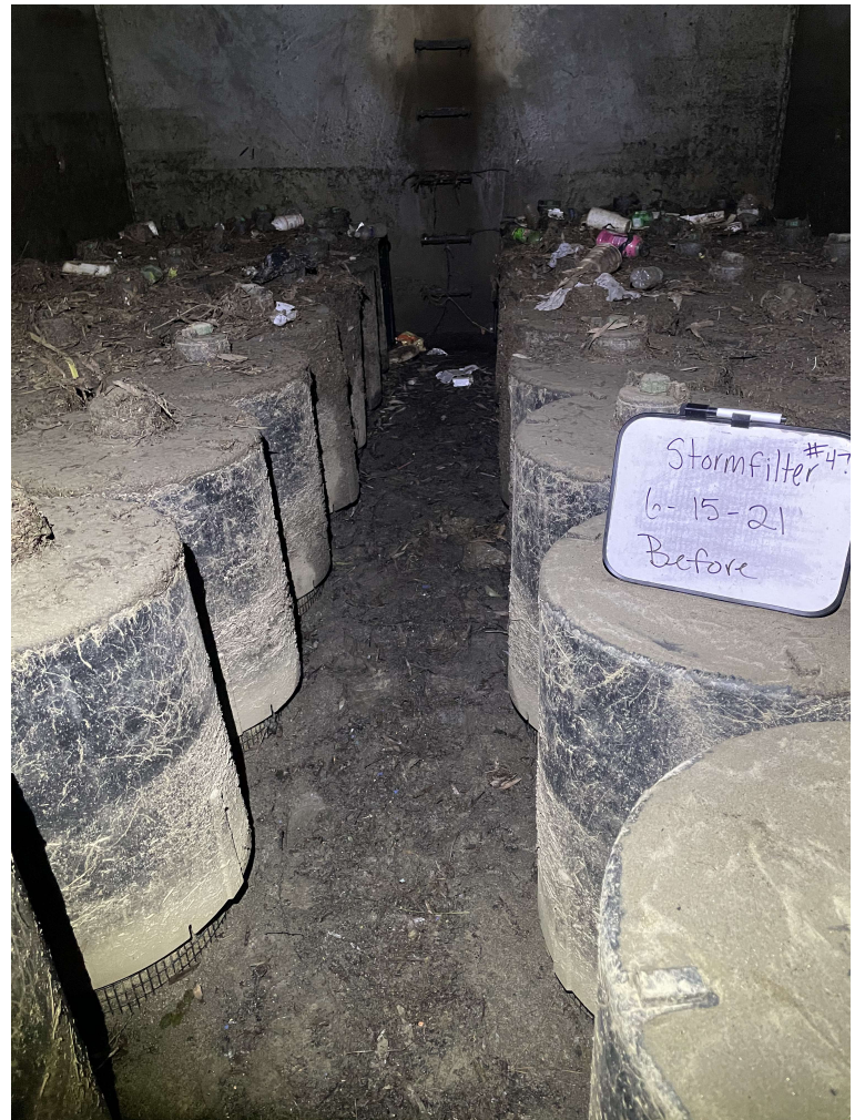
BMP 47 Stormfilter Before
