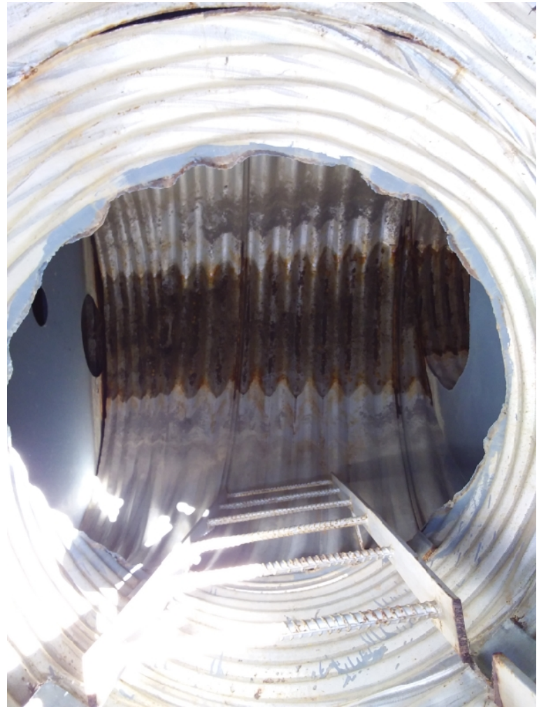
BMP 50- low flow orifice is clear
