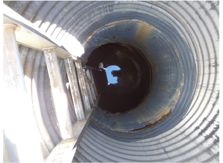
BMP 24: 7' of water standing inside- minimal sediment
