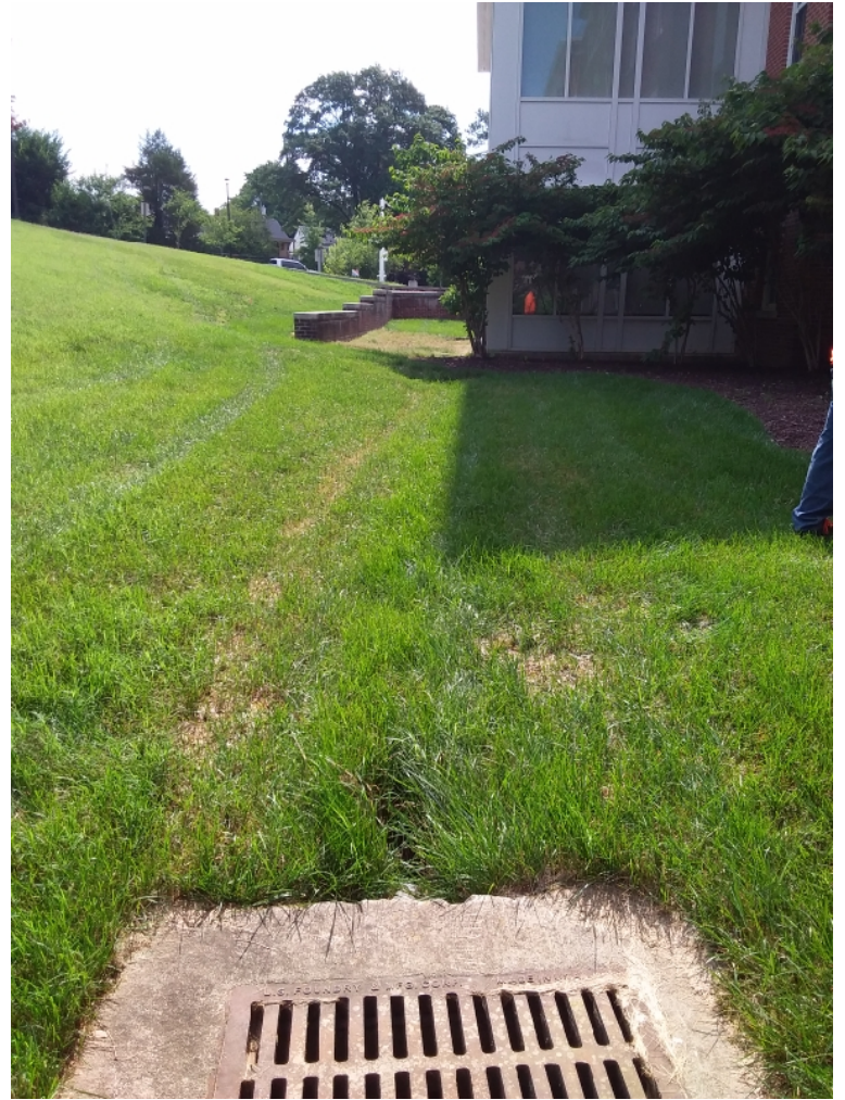
Noticed erosion and washout located SW of BMP 43
