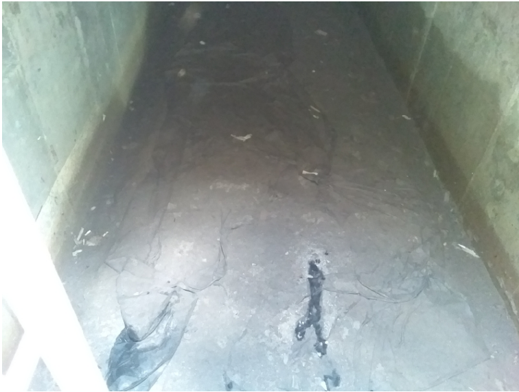
BMP 27- fabric needs to be re-positioned on sand filter side
