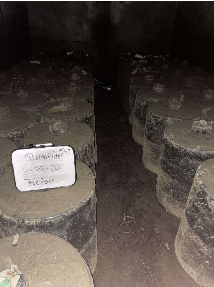
BMP 47 Stormfilter Before
