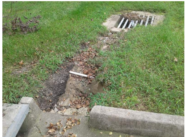
Unit 10: Major erosion to right of unit 10
