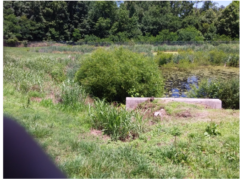
BMP 30- erosion occurring behind inlet structure and headwall that flows into forebay
