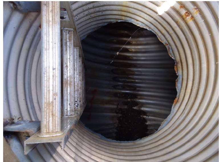
BMP 15: hardly any sediment at this access point
