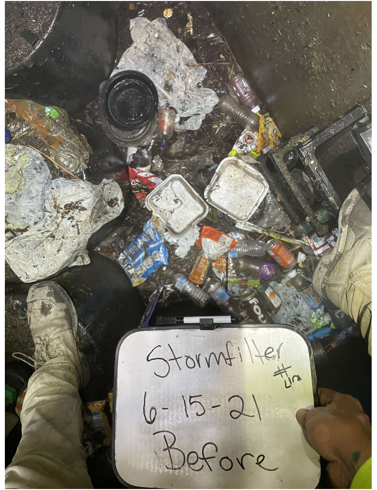
BMP 49 Stormfilter Before
