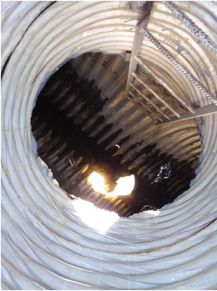
BMP 50- trace amounts of sediment
