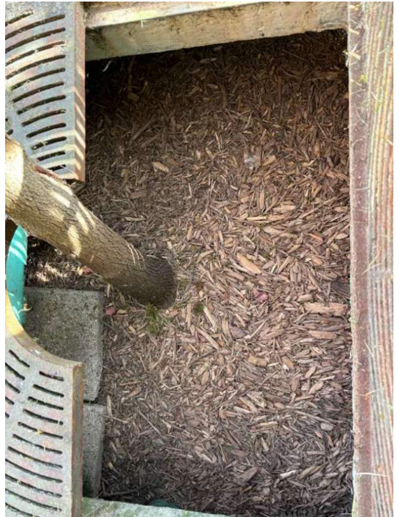
BMP 1- inside view after maintenance
