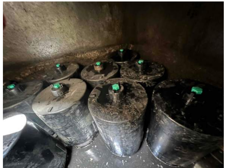
BMP 48- After replacing cartridges
