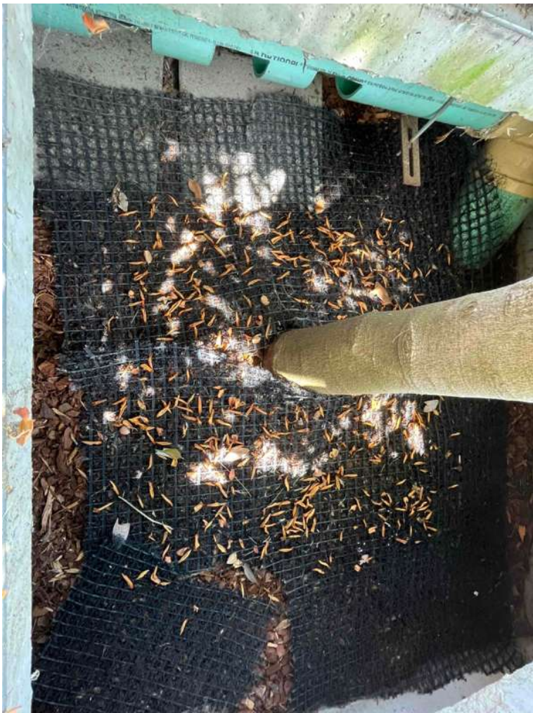
BMP 21- inside view after maintenance
