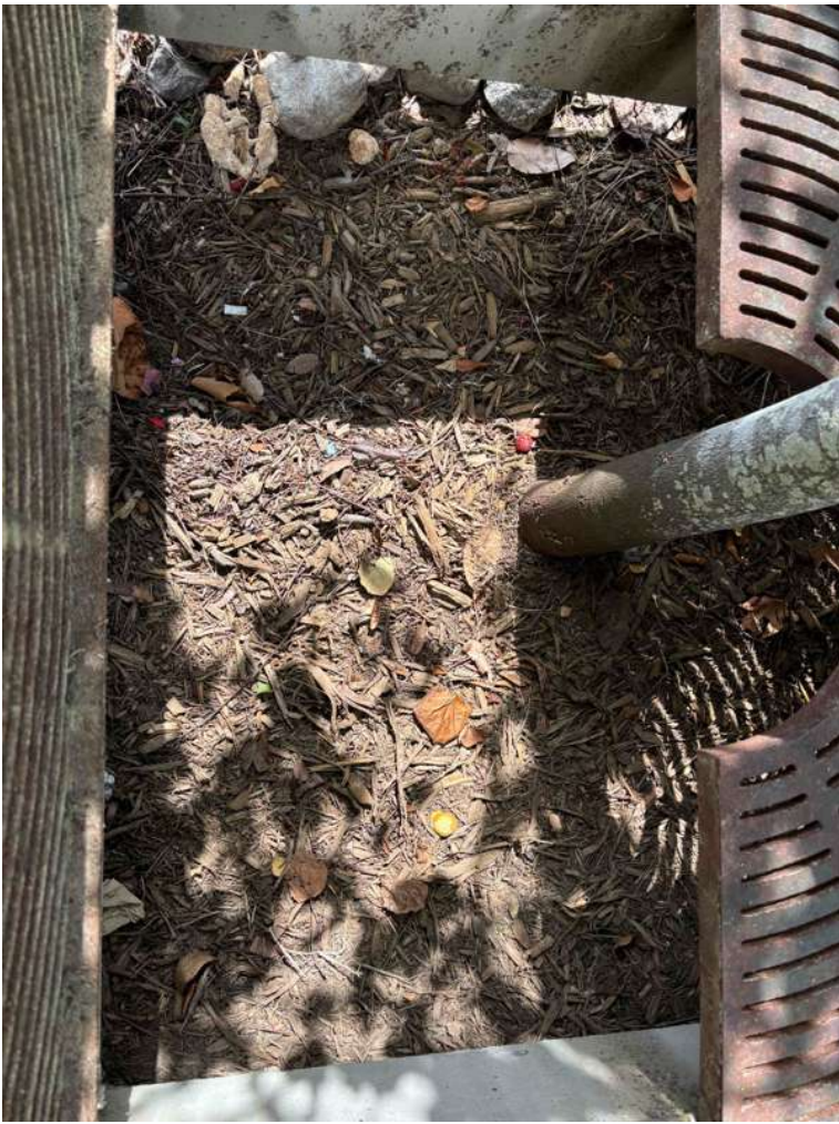
BMP 12- inside view after maintenance
