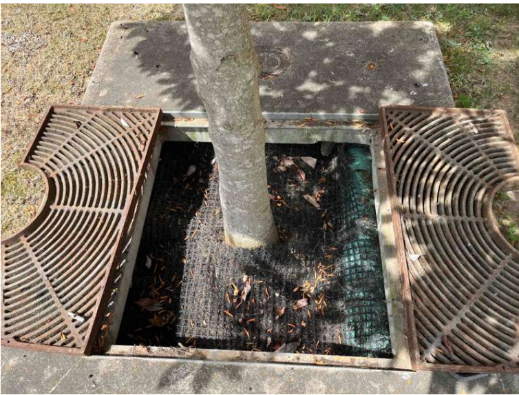
BMP 18- inside view after maintenance
