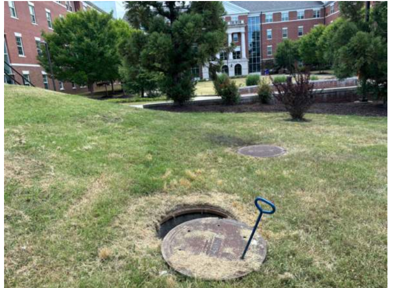
BMP 48- outlet chamber overall
