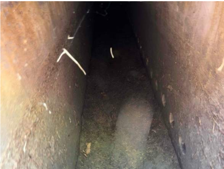
BMP 31- Sand filter side
