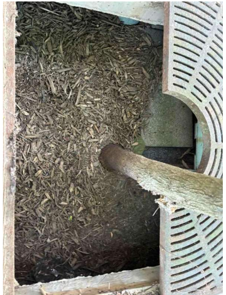
BMP 3- inside view after maintenance
