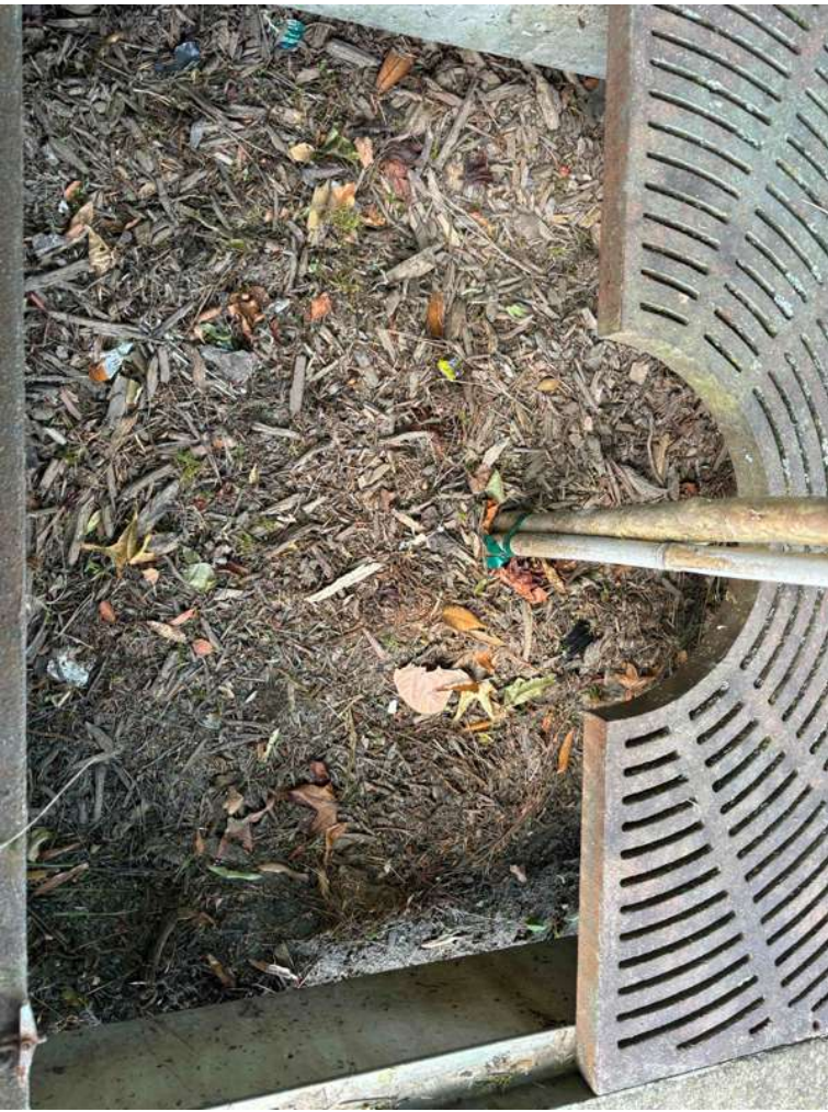
BMP 11- left inside view after maintenance
