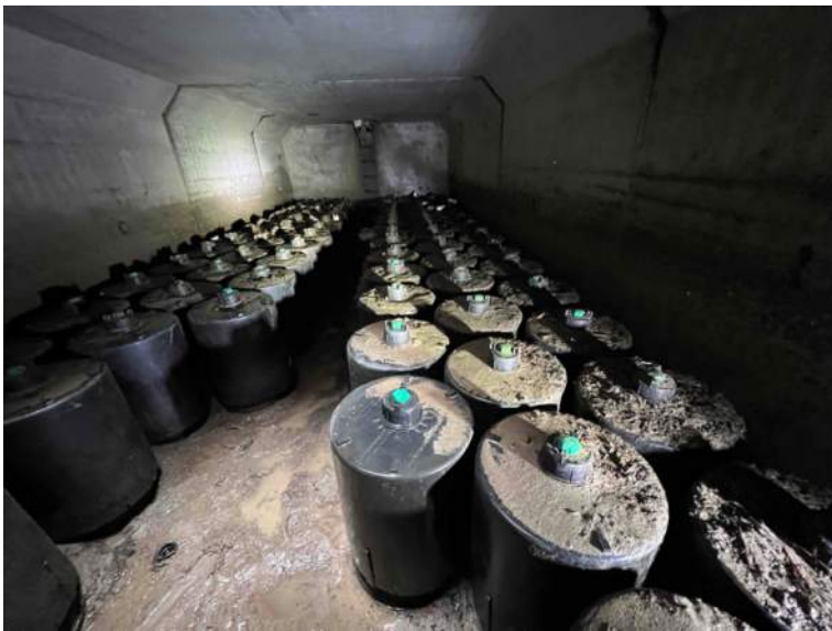
BMP 47 - after replacing cartridges
