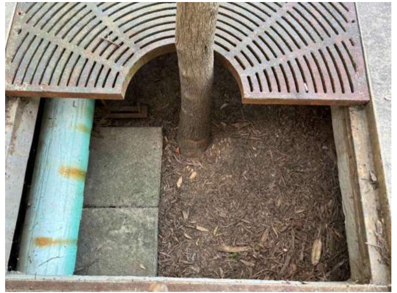
BMP 2- inside view after maintenance
