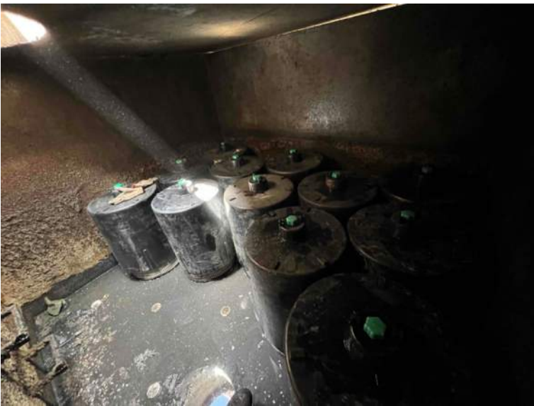
BMP 48- After replacing cartridges
