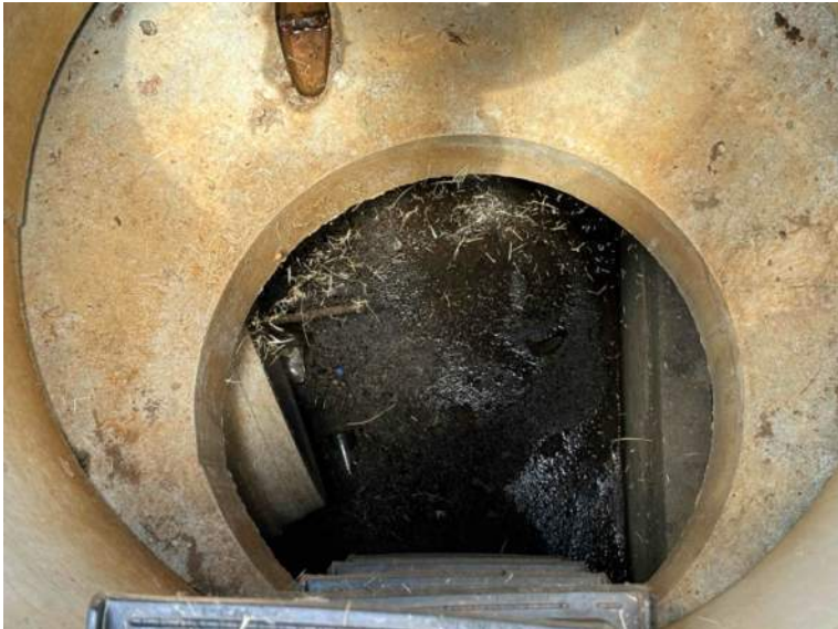
BMP 49- inside view of outlet
