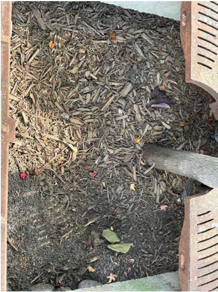
BMP 7- inside view after maintenance
