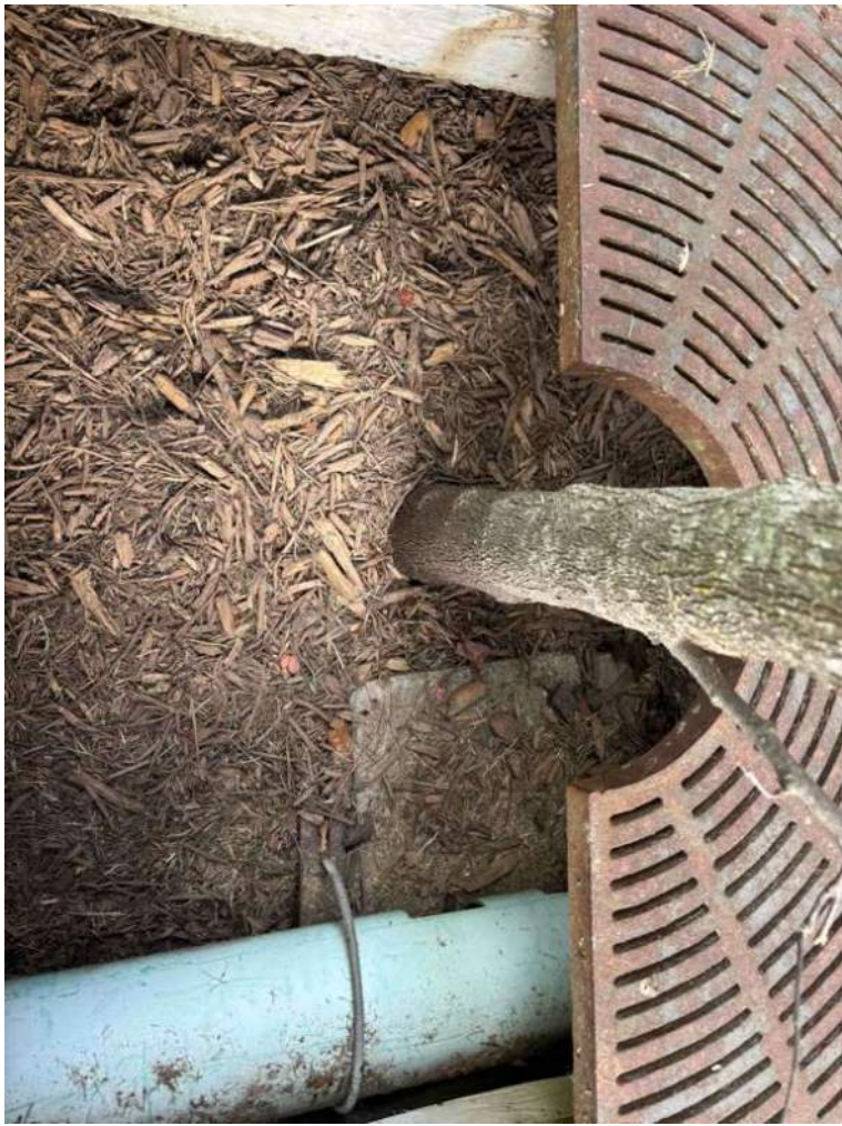
BMP 6- inside view after maintenance
