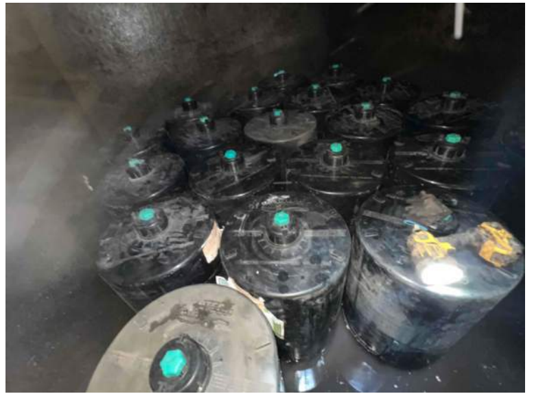
BMP 49 - after replacing cartridges
