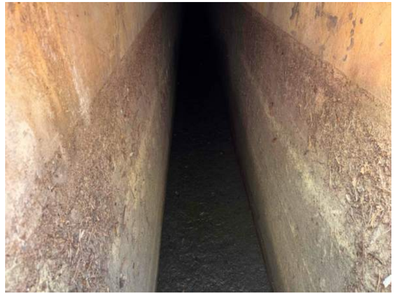
BMP 31- Sediment chamber
