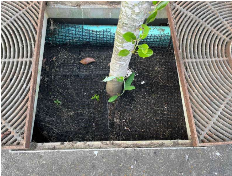
BMP 16- inside view after maintenance
