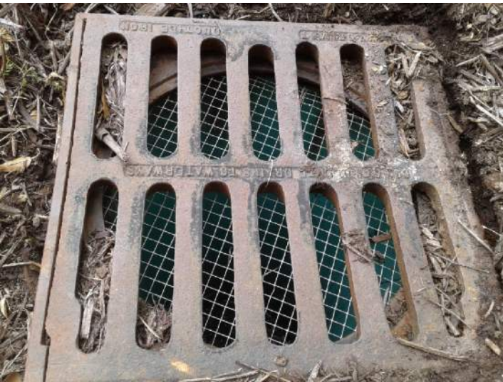
Unit 36. Screen installed. #1
