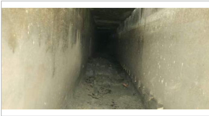
BMP 31 Sediment piles on top of sand filter (roughly 3-5" of sediment)
