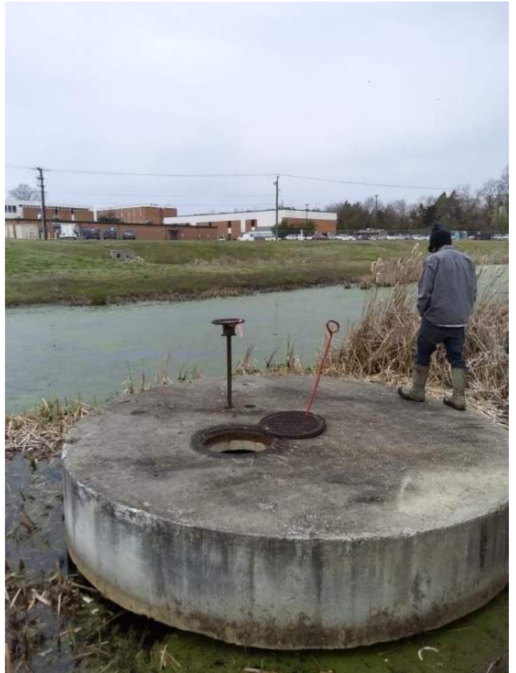
BMP 30: outfall structure
