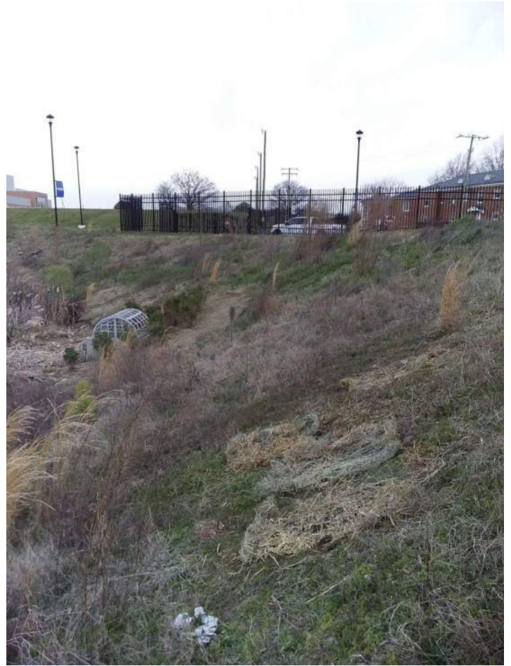
BMP 46: Small spots of erosion on side slopes near outfall structure were repaired with topsoil and then seed and straw matting was installed.
