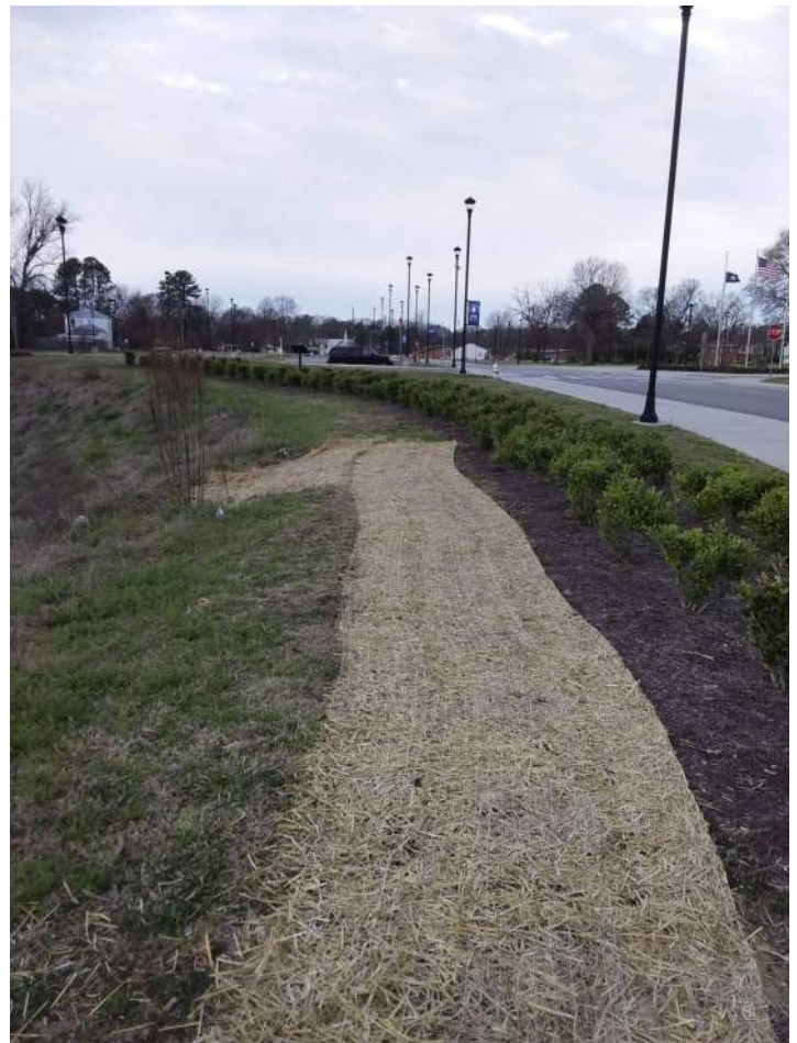
BMP 46: Erosion on the top of embankment repaired and then seed and straw matting was installed.
