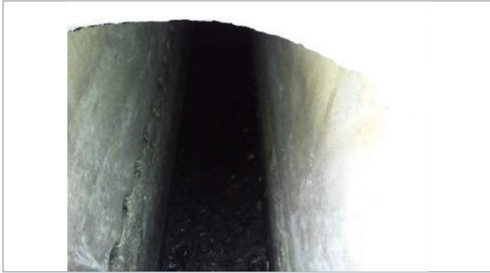
BMP 31: Sediment chamber facing south <1" of sediment in bottom
