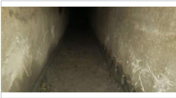
BMP 31 Beginning of Sand Filter, showing a thin layer of sediment on top of actual sand filter
