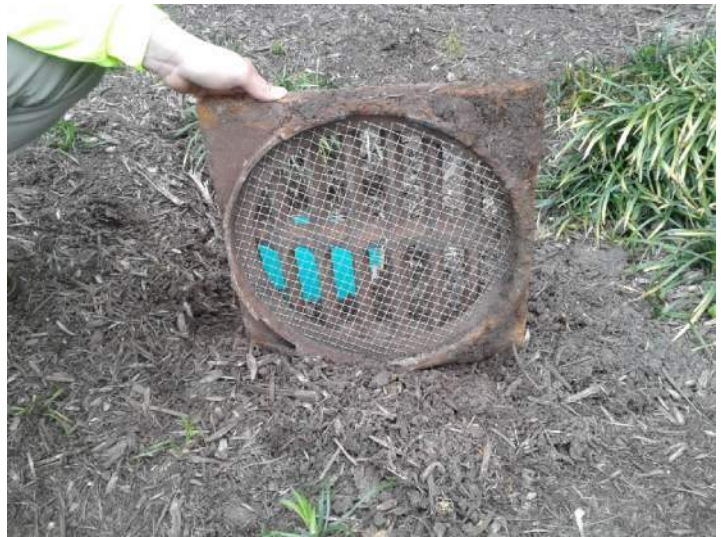
Unit 36. Screen installed #2
