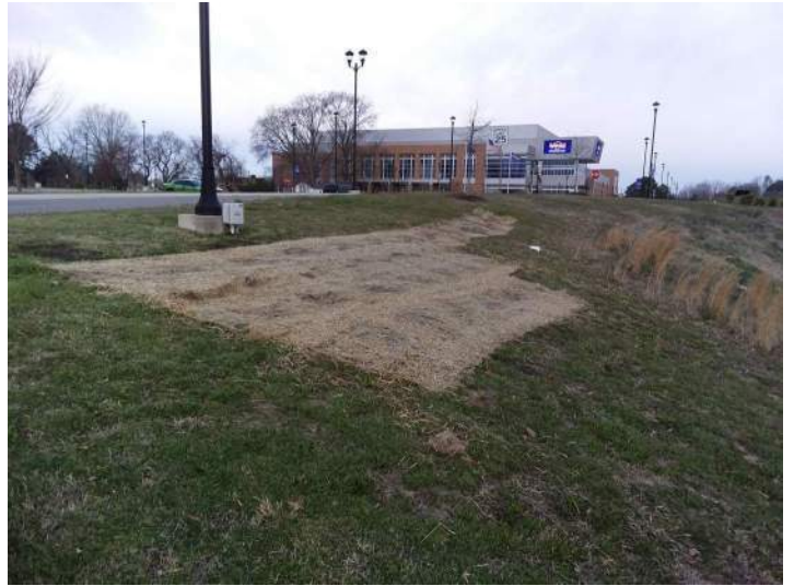
BMP 46: Side slope and top of embankment eroded area was repaired and stabilized properly.
