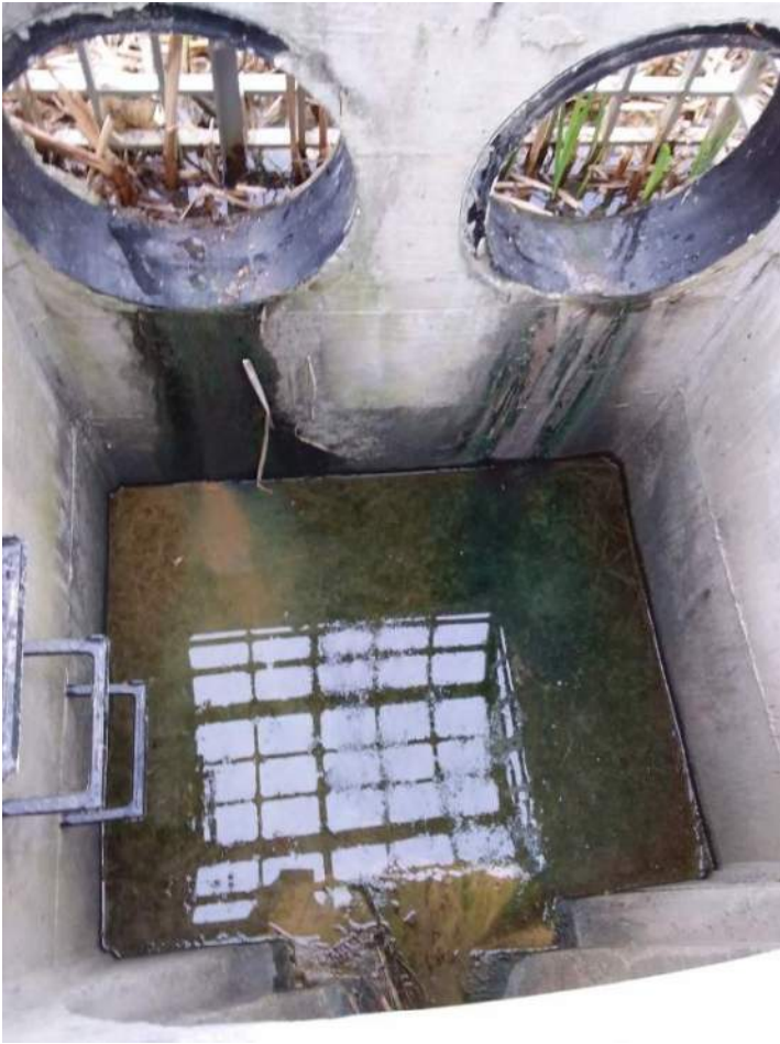
BMP 46: outfall structure with trash rack
