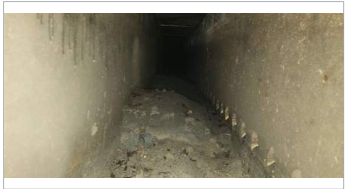
BMP 31 Continuing down the sand filter, showing more sediment piles.
